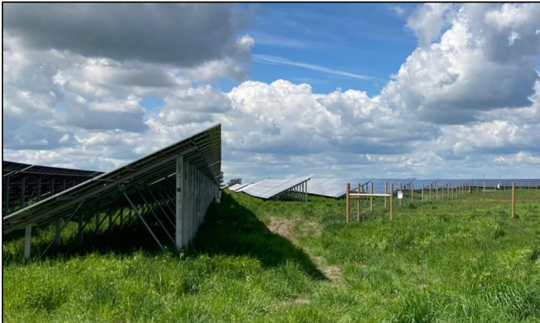
Plate 3.2 Example of a typical mounting structure
